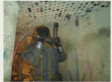
Proper PPE, specialized equipment, VIP International's experience and a joint venture attitude was attributed to the success of the repair.
