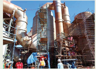
Minara's gas-to-gas exchanger is one of the largest of its type in the world with approximately 3,762 tubes and over 30 feet in length.
